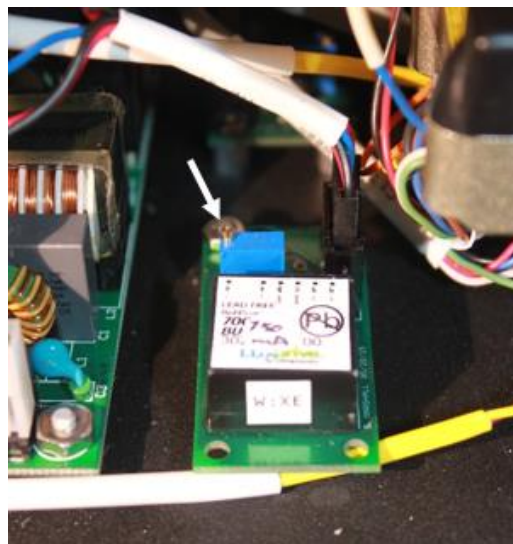
Figure 12: Lamp power supply showing potentiostat
